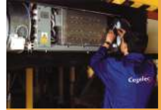
Static converter with DC and AC outputs
